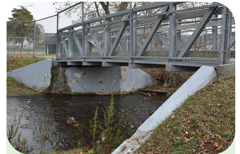
This bridge by the Jr./Sr. High School would be repaired to improve secondary entrance/exit.
